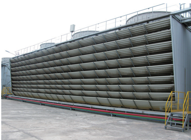
写真3 MS Indirect Cooling Tower
