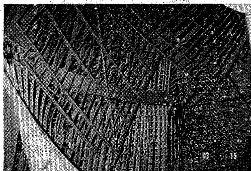
写真 4 脱落した充填材および破損した受梁 Photo.4 Excessive weight of scaling caused damages of fill supports and consequential destruction of fill arrangement
