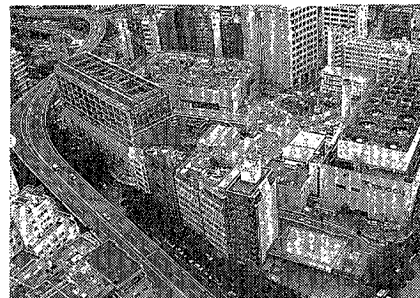
写真 5 新設（左上隅）、既設冷却塔（右上隅） Photo. 5 Cooling towers newly installed (top left-hand) and previously installed (top right-hand).
