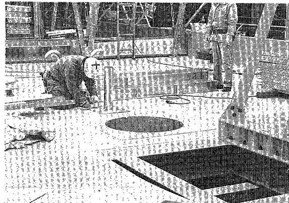
写真 5 冷却塔架台, FRP 切欠状況 Photo. 5 FRP being cut out at cooling tower supporting section
