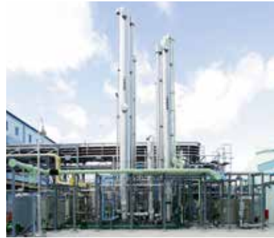
Biogas Upgrading System
